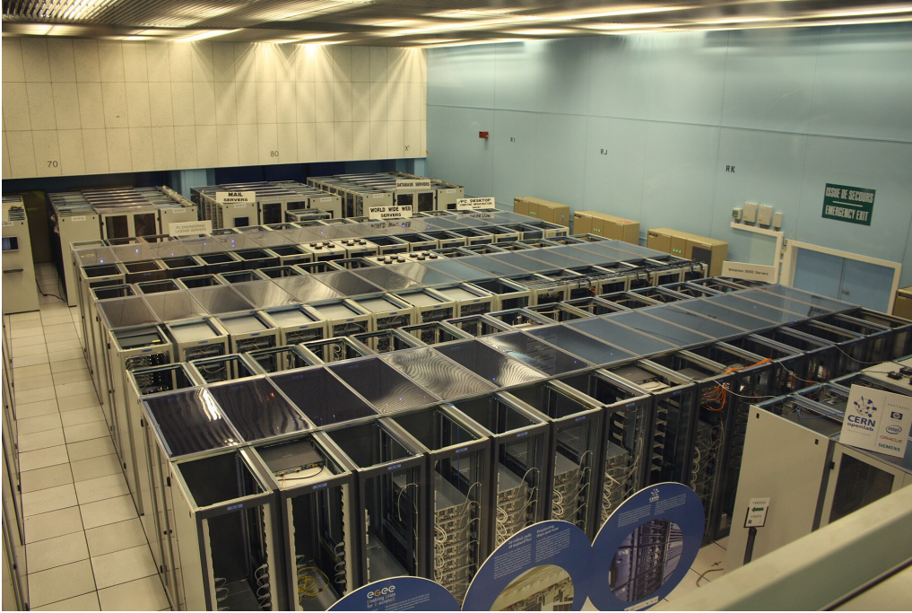
Figure 2.1: Example of a datacenter in CERN , Switzerland (2010) [19]. In the figure we can see servers within servers racks, and the network cables.
